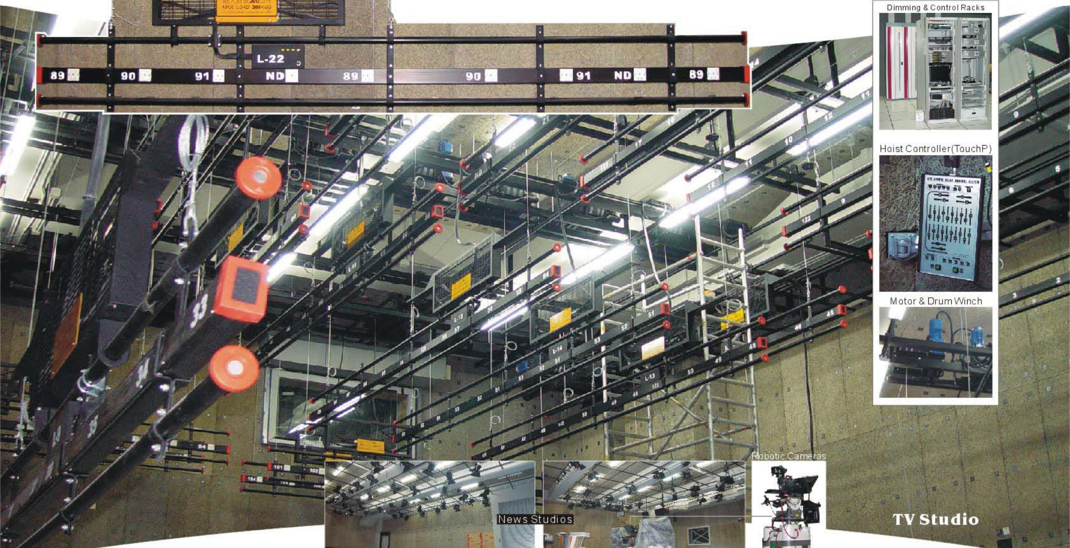
Dimming & Control Racks
