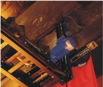
Motorized hoist system
