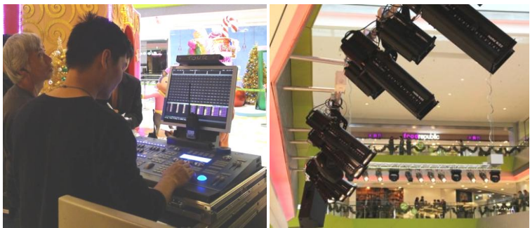
On-site lighting control by the lighting console.
