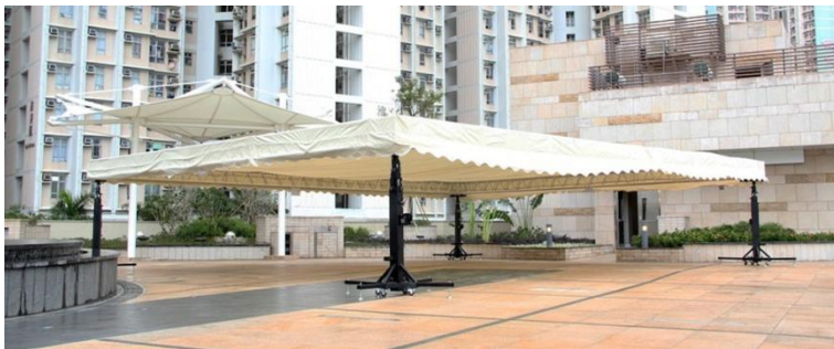
12m x 10m Truss Roof with Marquees supporting by 4 sets of 200kg Lighting Towers installed at L8 Rooftop Garden.
