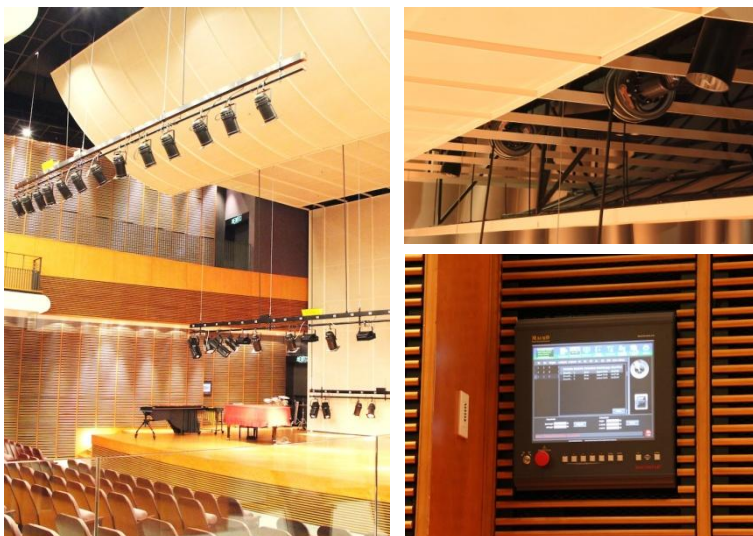
3 lightings bars are suspended from a metal construction, and can be raised up or lowered down by their own motorised winches via a MACHO hoist controller (bottom right). All winches drive the steel wires which pass through the pulleys mounted underneath the metal construction (top right) and then attach down to the lighting bars (left).
