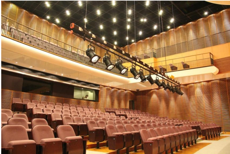
New motorised lighting bar mounts the existing front of house lighting fixtures, which provide localized light spots for the stage.
