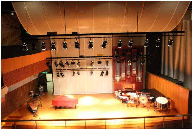
New lighting fixtures were upgraded at the centre of the stage, providing a general wash of the whole performing area.
