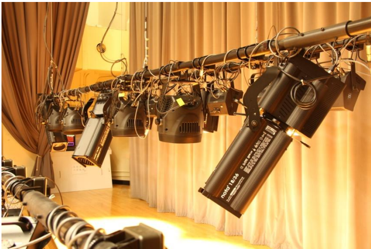
Over 75% of the stage lighting fixtures were upgraded with LEDs.
