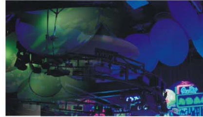
Motorized Lighting Truss and fixtures
