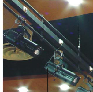
Motorized Lighting Suspension System with stage fixtures
