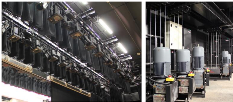
All stage lighting fixtures were installed on motorised lighting bars lifted by MACHO drum winches.
