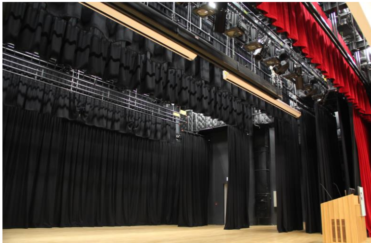
Stage features Gerriets red curtains and JD McDougall black curtains with automatic control.
