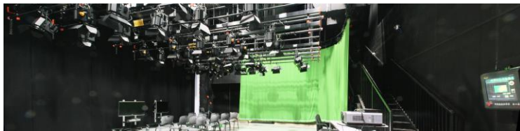
Specifically dyed chroma-key green cyclorama, which is set at one side of the VPS. All lighting fixtures are installed on the motorised lighting bars at the centre of the studio, providing professional lighting for shooting.
